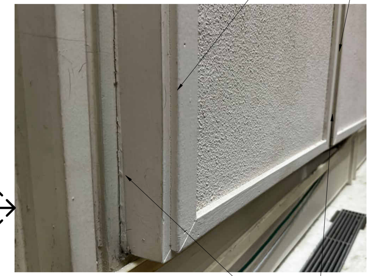
BASE BID: PRIME AND PAINT EXISTING ACOUSTIC PANELS AND WOOD FRAMES AND TRIMS. (TYPICAL FOR ALL PANELS ON NORTH, SOUTH AND EAST WALLS)
