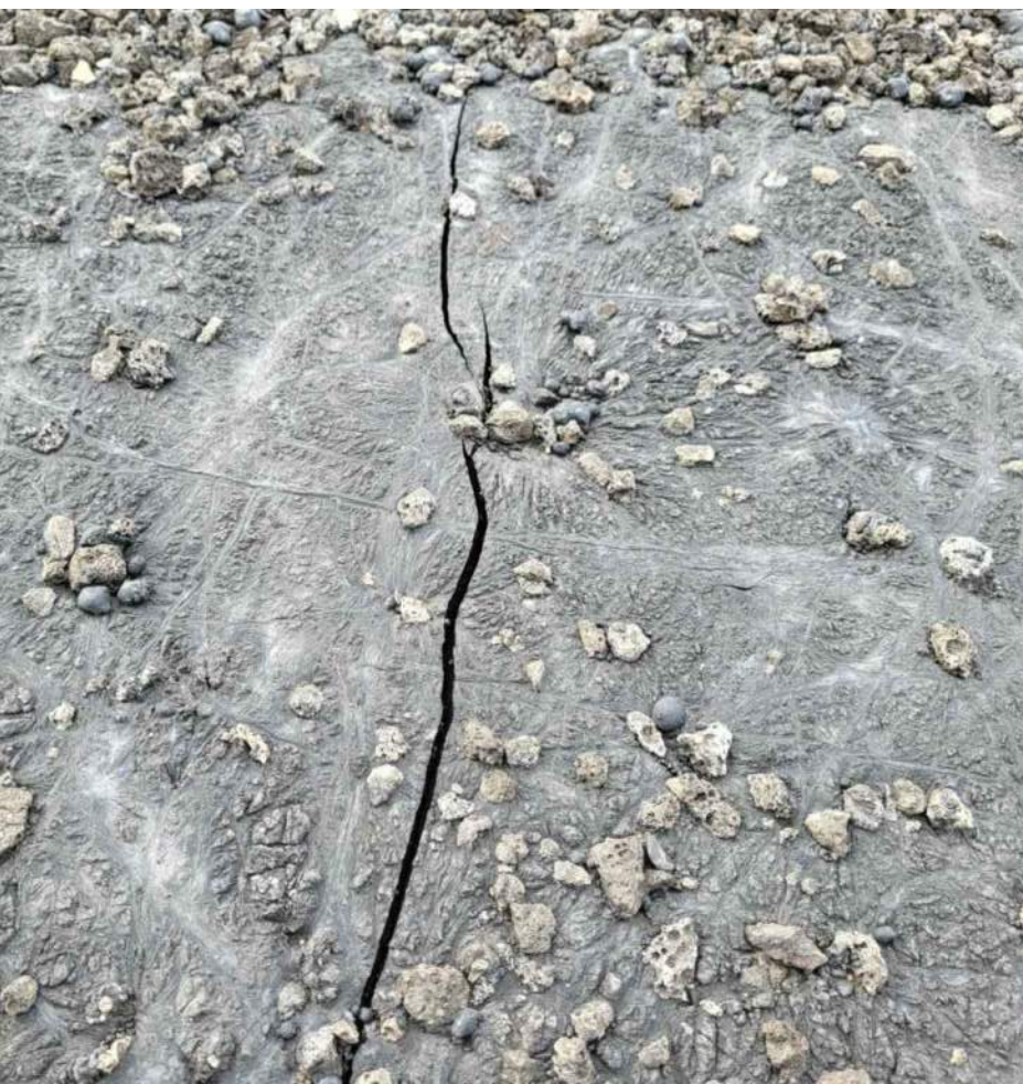
CURRENT CONDITION - TEARS AT ROOF A
