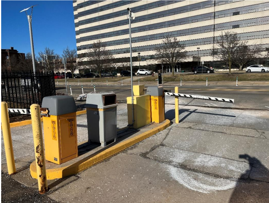
Photo 29: Lot 70 (note wireless connectivity on this lot)
