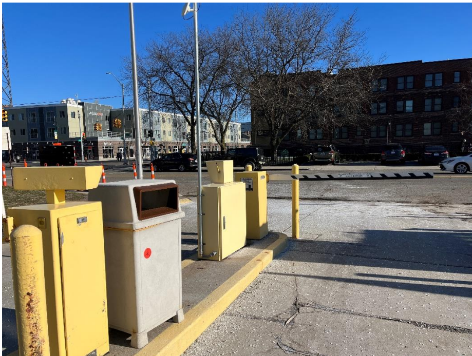
Photo 30: Lot 71 (note wireless connectivity on this lot)
